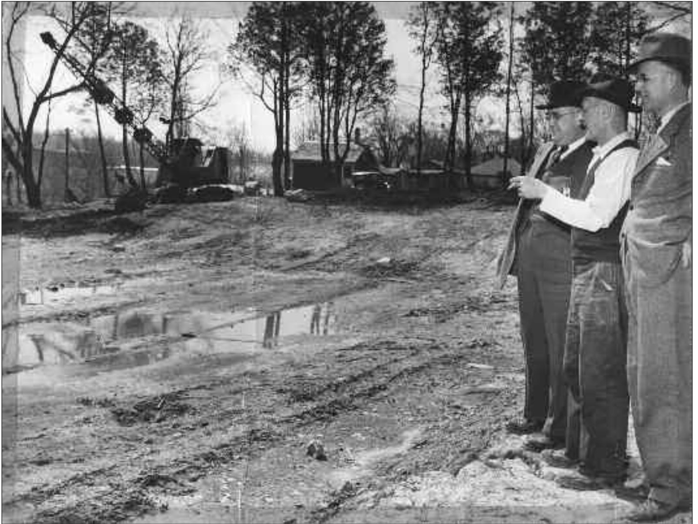
1509 Fundraising chair F. Adair Campbell (left) and construction supervisor Dave Eizerman (centre) are on hand as excavation begins on Blenheim Street, just east of Nelson Street, for construction of the Lions Club swimming pool in 1948. The man on the right is possibly Alvin Jordan.
